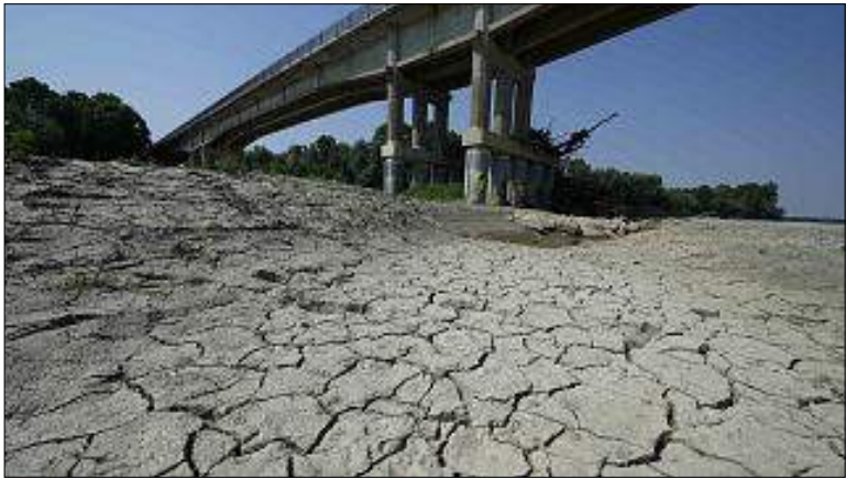
Dry cracked land is visible under a bridge in Boretto on the bed of the Po river
